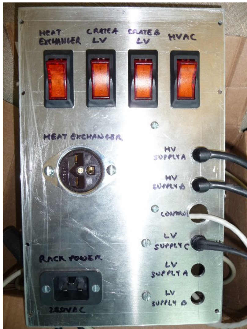
Figure 4.21: TALE Breaker Panel. The HiRes-II panel was composed of GFCI breakers, which frequently tripped when HV power was enabled to the cameras. The new unit (pictured here) is composed of a series of standard over-current breakers and control relays. The internal relays in the breaker panel allow the power control board to determine when HV and LV supplies are provided power.
