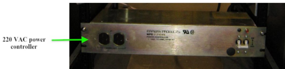
Figure 4.20: 220 V Power Controller. This is a picture of a 220V Mapway power controller module. 220 V power is switched by external power board control lines connected to an internal relay on the control module.
