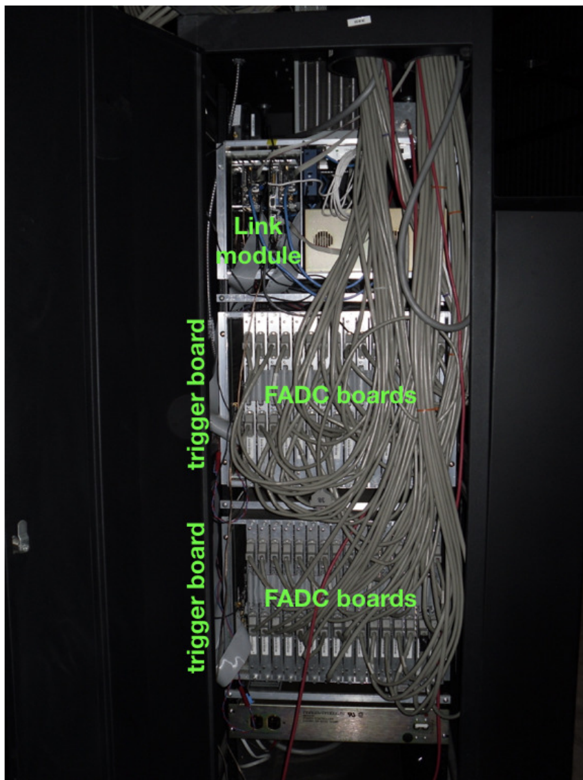
Figure 2.17: Photo of front side of TALE electronics rack.
